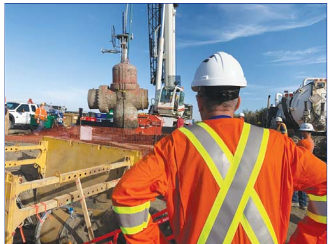
Above: A worker looks on during removal of a valve south of Morden.
