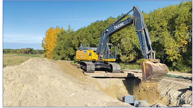
Above: Once the cap is in place, backfilling of the excavation begins.
