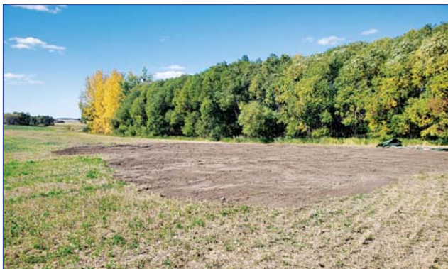
Above: With backfill completed and the topsoil replaced, the land is ready to be returned to its pre-construction state.
