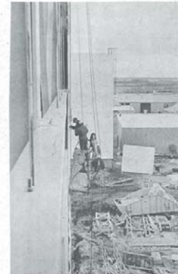
Workmen are seen here closing in the huge main building for the refinery and load-out facilities.
