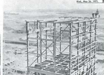
A mining tradition was observed at this evergreen was planted on the highest place piece of steel at the top of the hoisting headframe.
