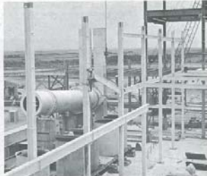
Steel columns for the refinery. A section of the product dryer at left resembles a gun barrel.
