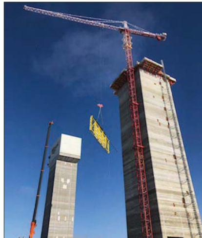
Work is underway on the superstructure at the top of the south headframe at the K3 expansion.
