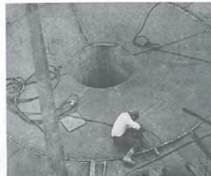
A welder is seen here at work on the interior of the hot thickener in the refinery.
