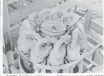
A cluster of cyclones used for separating solids from liquids, just one of many processes at the Sylvite refinery.
