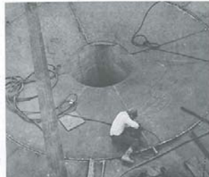
A welder is seen here at work on the interior of the hot thickener in the refinery.
