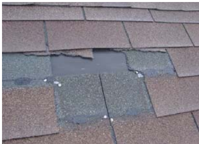
Are your roof shingles disintegrating? Moss is growing on them? Make an appointment with a roofing expert.
